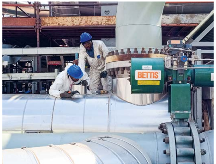
Technicians secure aluminum jacketing on insulated process piping, ensuring full compliance with international thermal performance standards.
