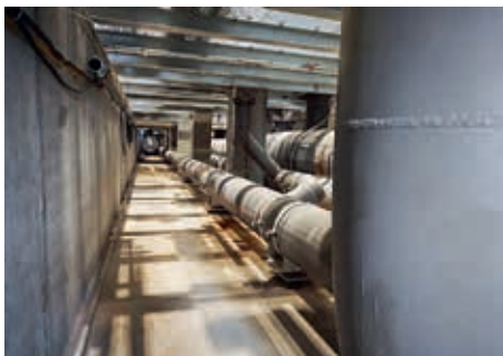
With a length of almost 50 meters, the pipe network runs in the plant’s basement, supplying the process with wastewater and coolant.
