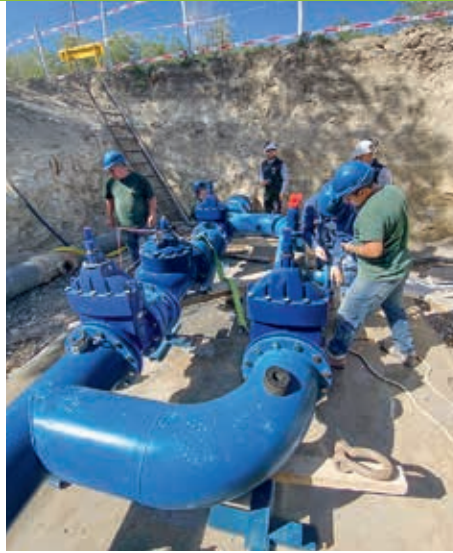
The DN 300mm pressure reducing station will connect the main reserve to a secondary reserve in Puerto Madryn.
